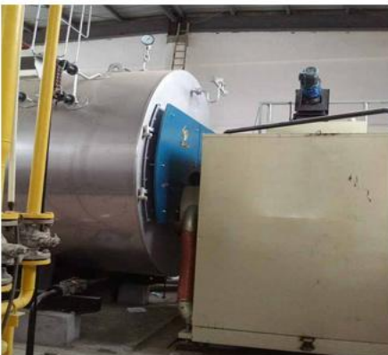
8 tons biomass steam boiler
