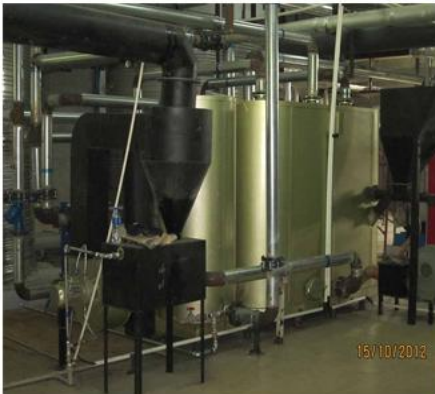
1.2 million kcal supporting water heater
