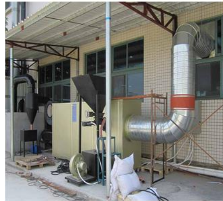
900,000 kcal matching hot blast stove
