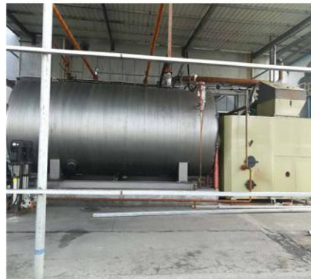
10 tons hot water boiler
